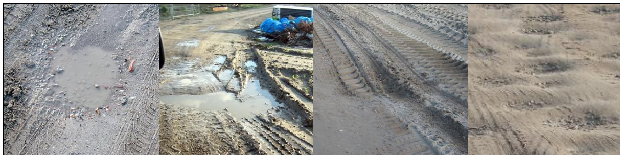
Figure 55: examples of damage to an unpaved road.
