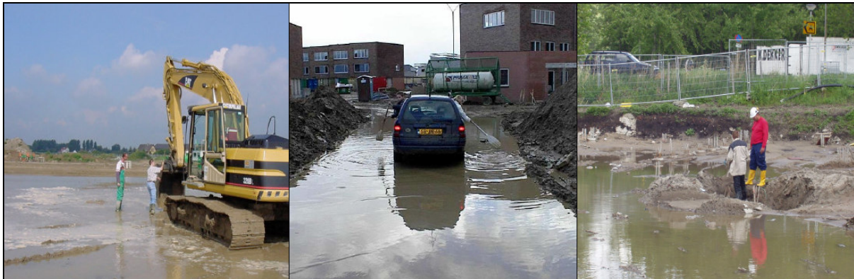
Figure 75: water logging on construction sites.
