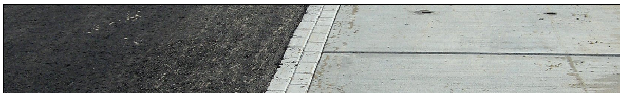
Figure 58: combination of concrete plate and asphalt pavement as temporary road on Duyfrak.
